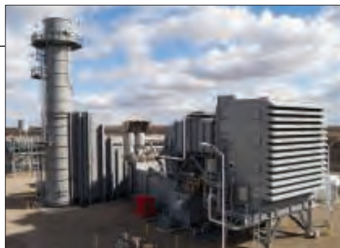
FIGURE 3. The modern aero-derivative gas turbine installation shown here includes a 100-MW gas turbine. The inlet air system, gas turbine and exhaust gas system are also shown
