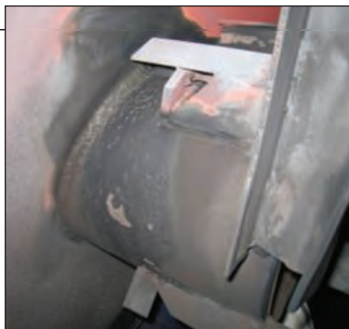
FIGURE 4. The effects of two-phase FAC are shown here in a deaerator
